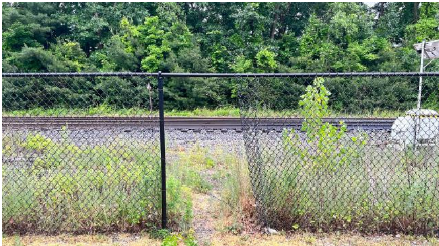
Figure 3-5. Damaged Fencing South of Broadway
