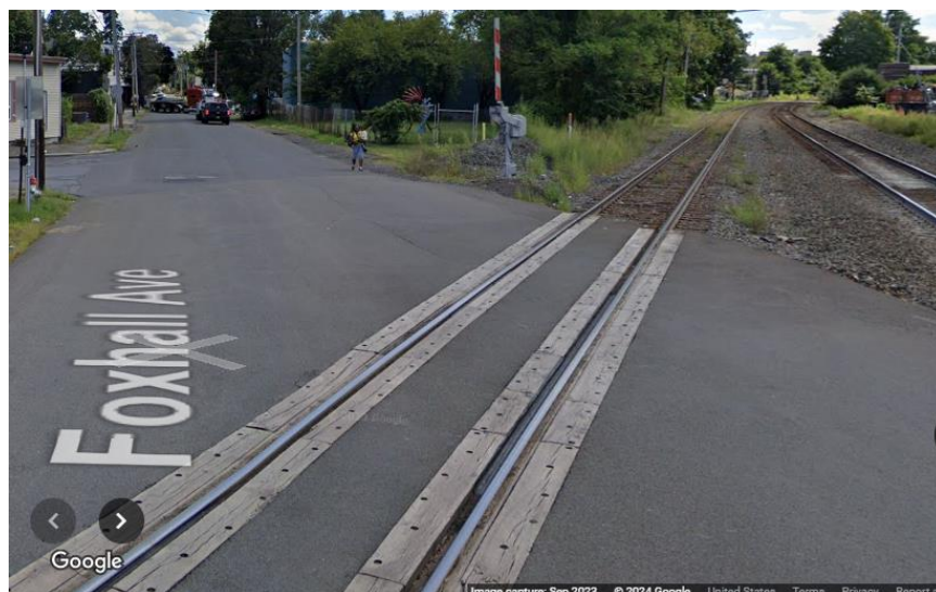
Figure 5-16. Lack of Pedestrian Sidewalk at Foxhall Ave.
