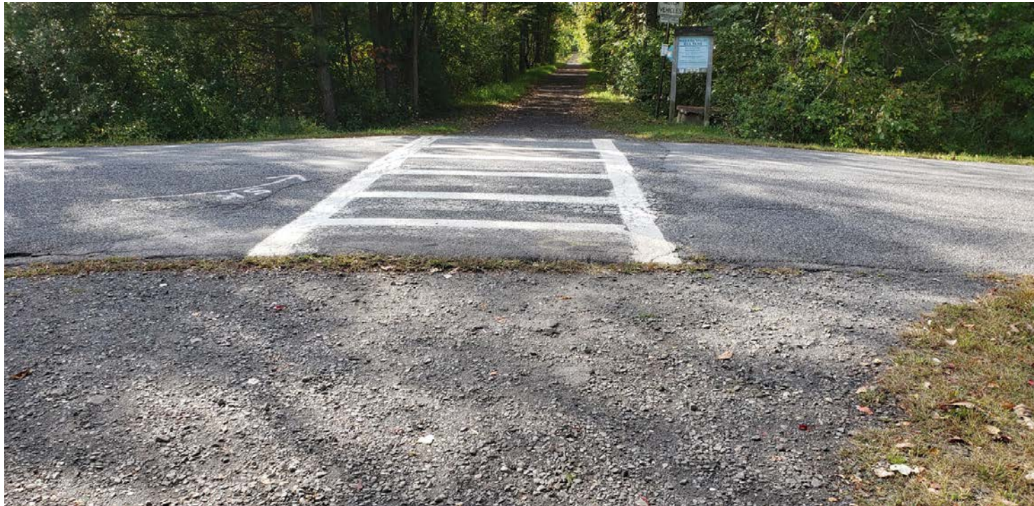
Significant change at path and roadway intersection at Huguenot Street
