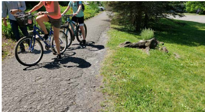
Broken and deteriorated asphalt results in rough and uneven pavement.
