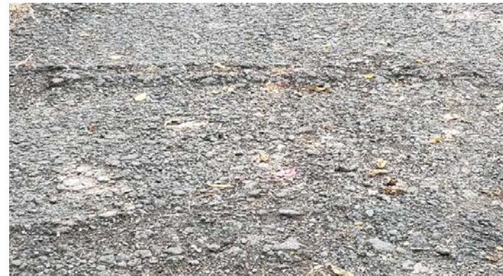
Broken and deteriorated asphalt are compounded by areas of trail surface pushed up the tree roots that occur unexpectedly along the trail.
