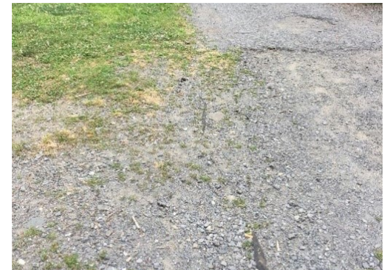
Deteriorated surface adjacent to Main Street crossing
