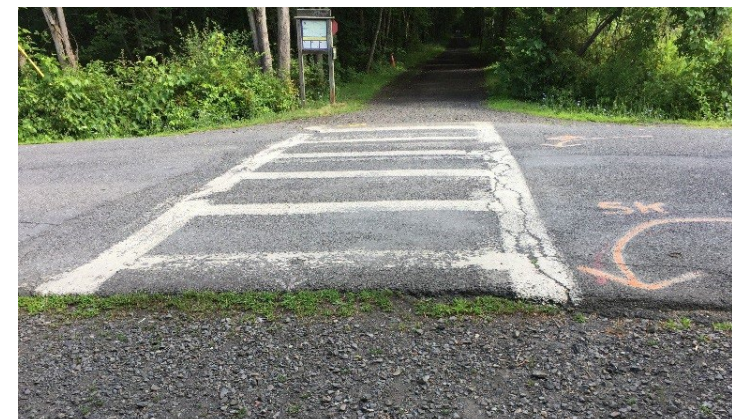
Vertical discontinuity at road crossing
