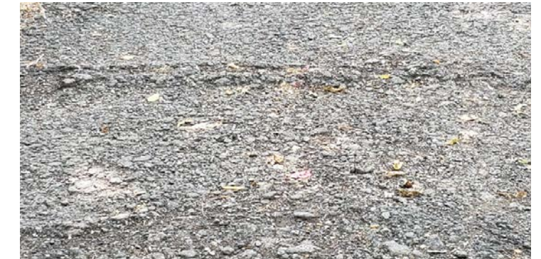
Broken and deteriorated asphalt are compounded by areas of trail surface pushed up the tree roots that occur unexpectedly along the trail.
