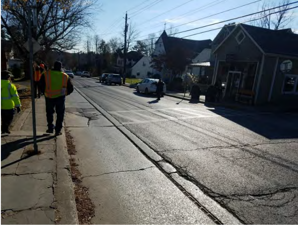
Photo 3: Poor pavement condition in area where trench drain is present.
