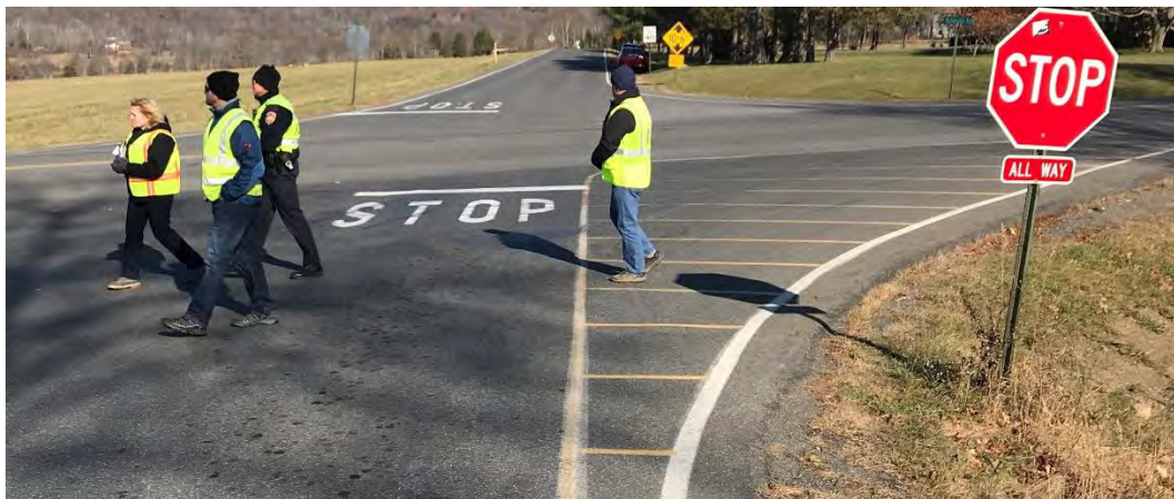
Photo 9: Faded yellow channelized crosshatch markings on NYS Route 299 at Butternville Road.
