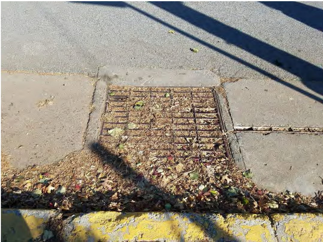
Photo 8: Drainage structure full of debris near Maple Lane.
