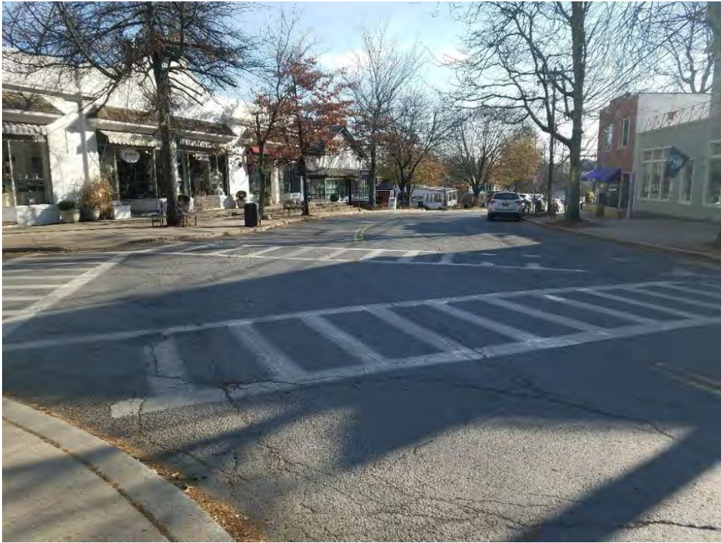
Photo 1: View of faded pavement markings and diagonal crosswalks at Rock City Road.
