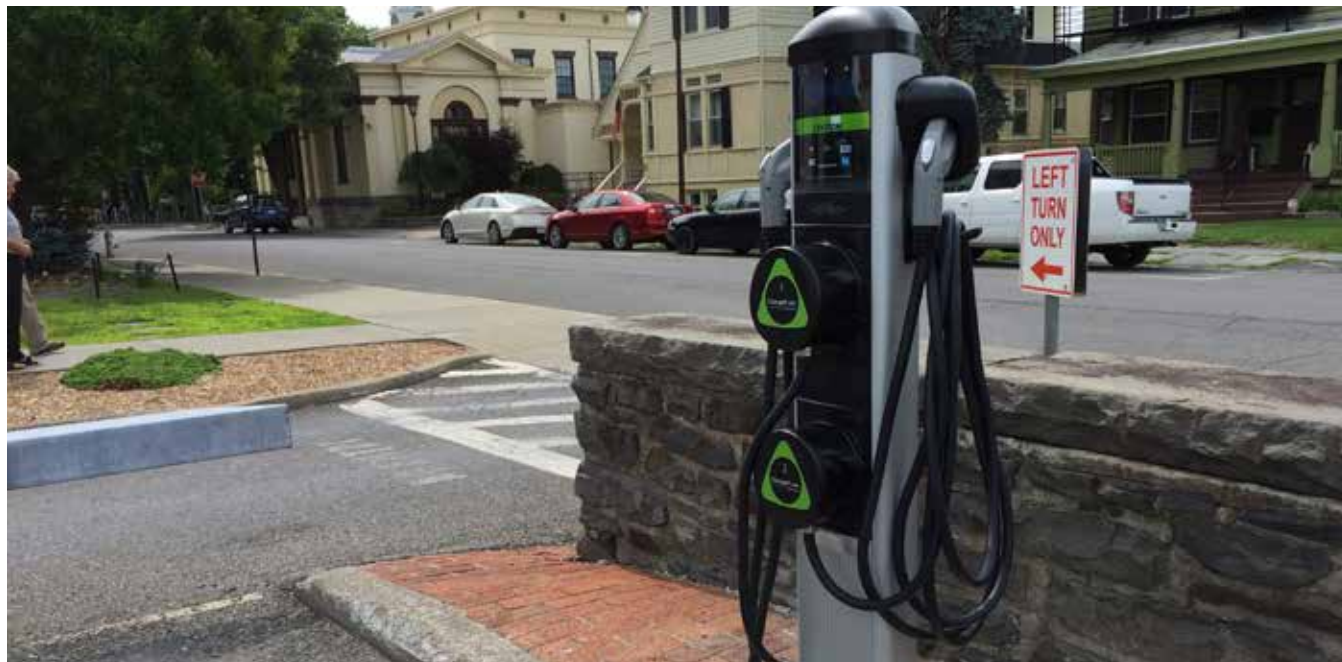
Electric Vehicle Charging Station at the Ulster County Office Building.
