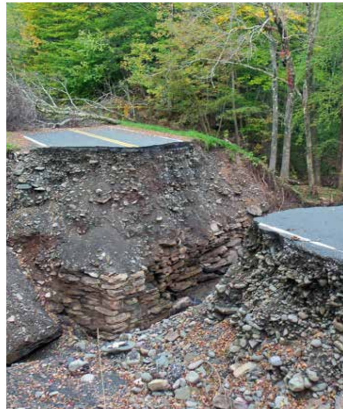
Washout damage from Hurricane Irene, Shandaken. Daniel Case
