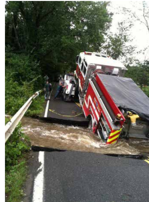
Firetruck being rescued by tow truck from culvert that has collapsed due to severe flooding.
