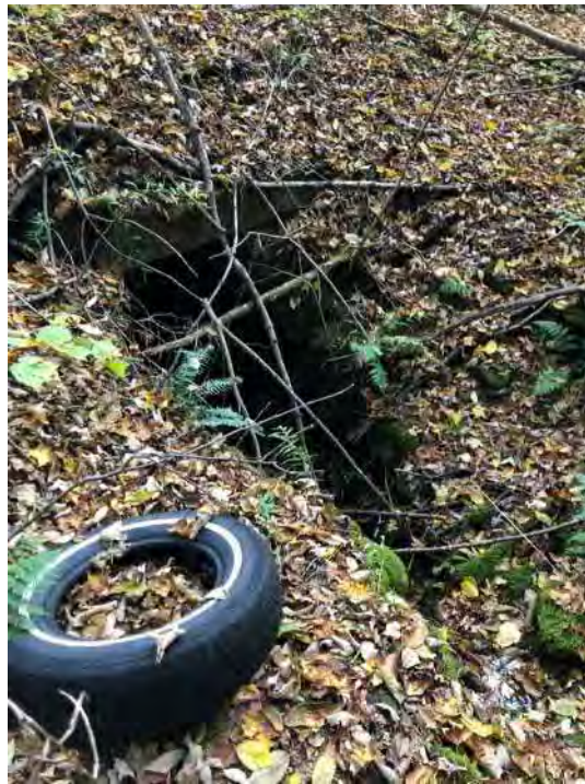
Photo 20. Stream 10 culvert inlet and tire debris.
