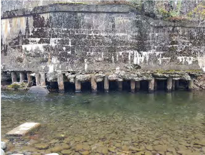
Figure 2-13: West abutment deterioration due to scour
