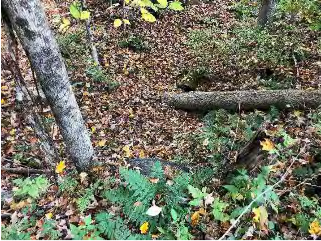
Photo 7. Steel pipe culvert under rail – no evidence of hydrology/stream, inlets or outlets identified.
