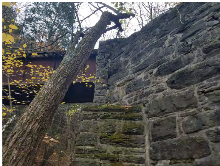
Figure 2-8: Separation beginning at the joint between the cheekwall, backwall, and northwest wingwall at the West Abutment
