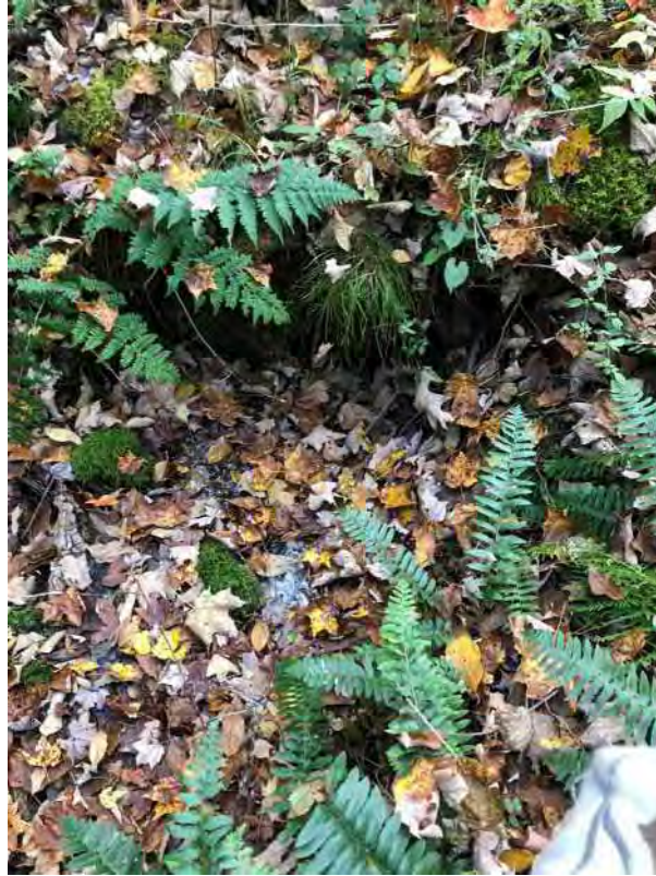
Photo 19. Stream 9 – leaf clogged culvert inhibiting flow.
