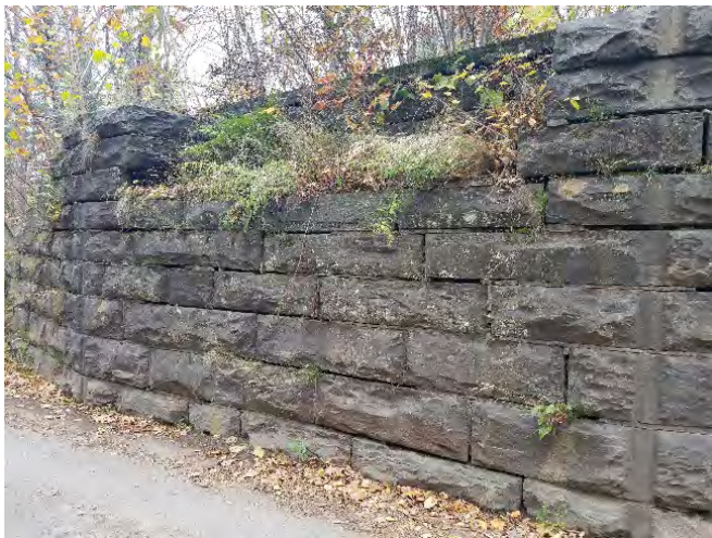
Figure 2-11: Deterioration of the grout between the stone blocks
