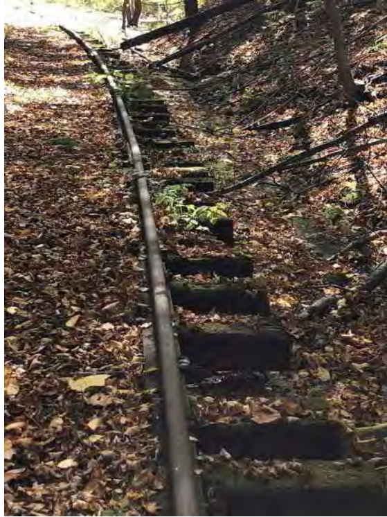
Photo 29. Stream 3 partially undermining tracks to right.
