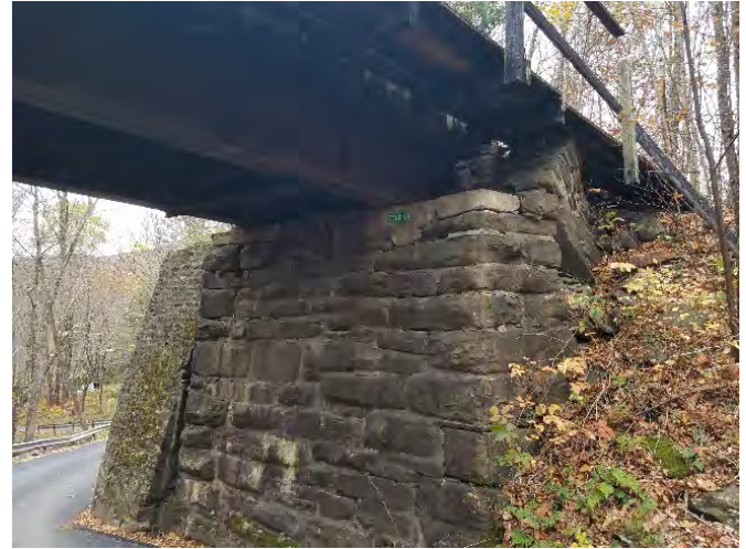
Figure 2-5: Displacement of East Left Wingwall
