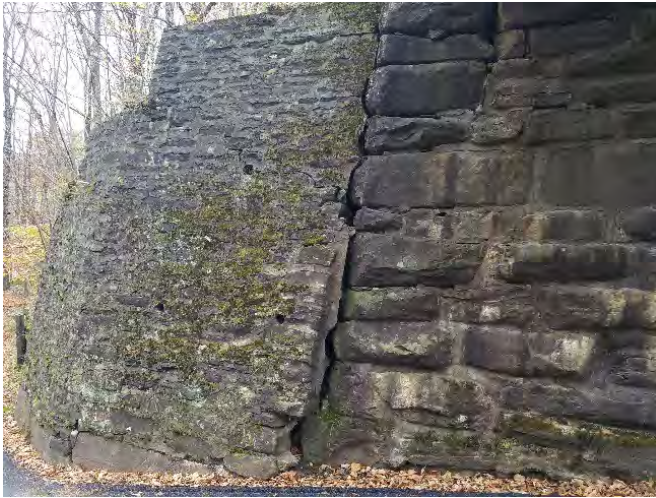
Figure 2-4: Separation between East Abutment and Right Wingwall
