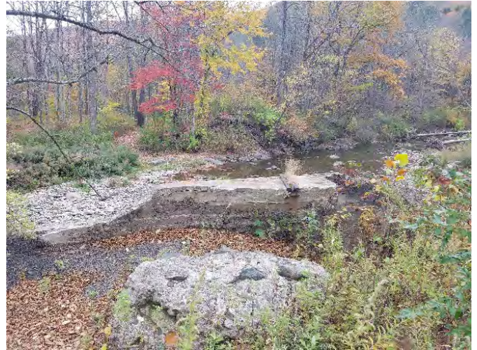
Figure 2-14: Looking east toward missing east abutment
