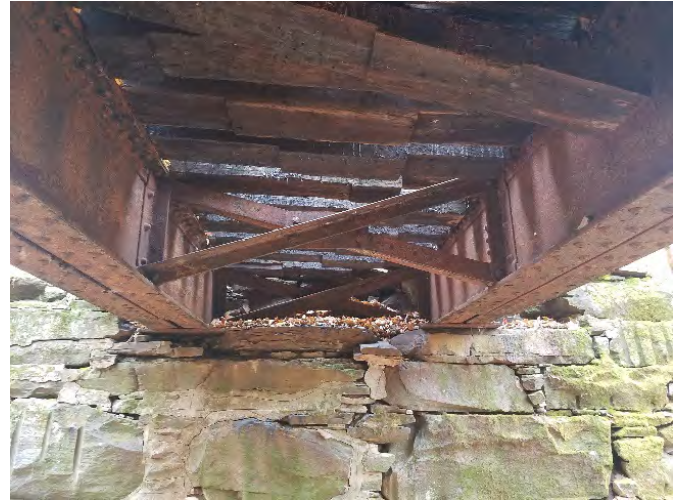
Figure 2-16: Deterioration at the bearing area of the east abutment #2
