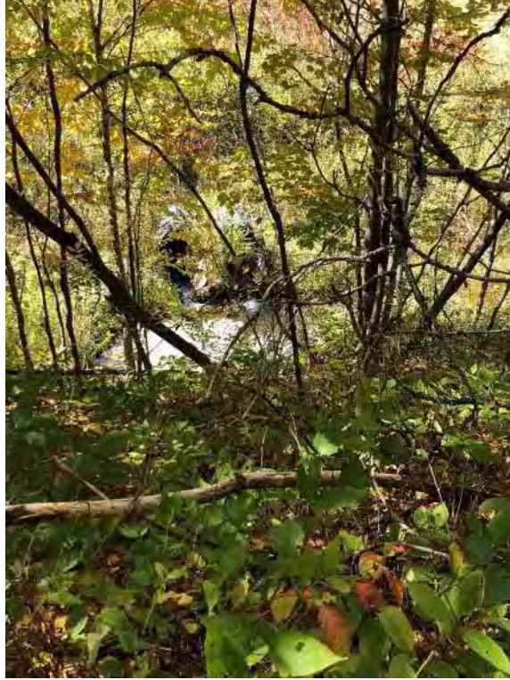
Photo 31. Stream 4 from top of railroad embankment – note double culvert enters separate culvert under railroad.
